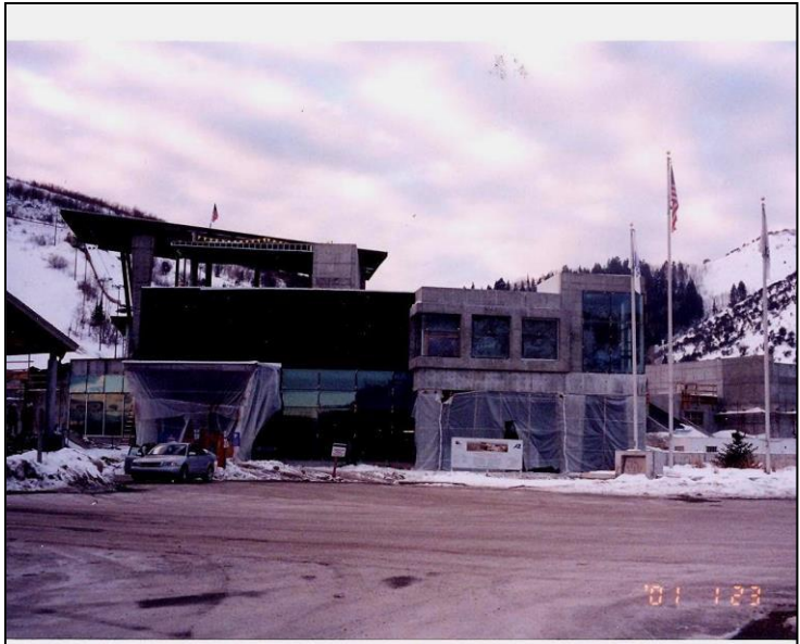
Joe Quinney Winter Sports Center / Alf Engen Ski Museum under construction, January 23, 2001
